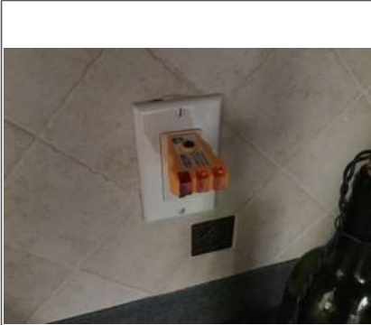
Outlet to left of sink does not work
